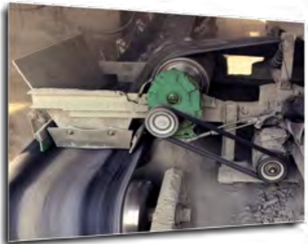
.....> Belt conveyor drive
